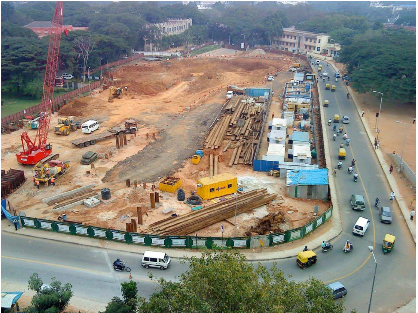
Aerial View of Sir M. Vishveswaraya under Ground Station Works (Central College)
