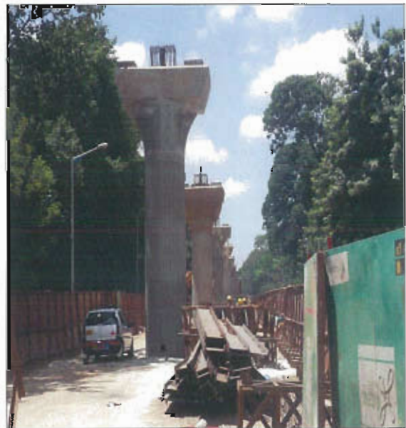
The completed Piers stands in the MG Road ready for segments launching
